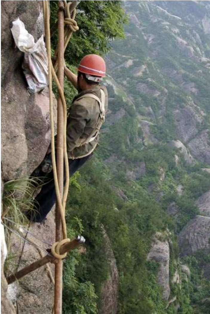
Yu Ji takes charge of the most dangerous part of the project - drilling the holes to set up pipes to support the footpath
